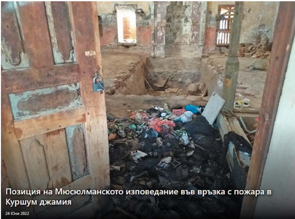
Figure 1: A photograph showing the interior of Kurshun Mosque in Karlovo taken after the fire. 5
