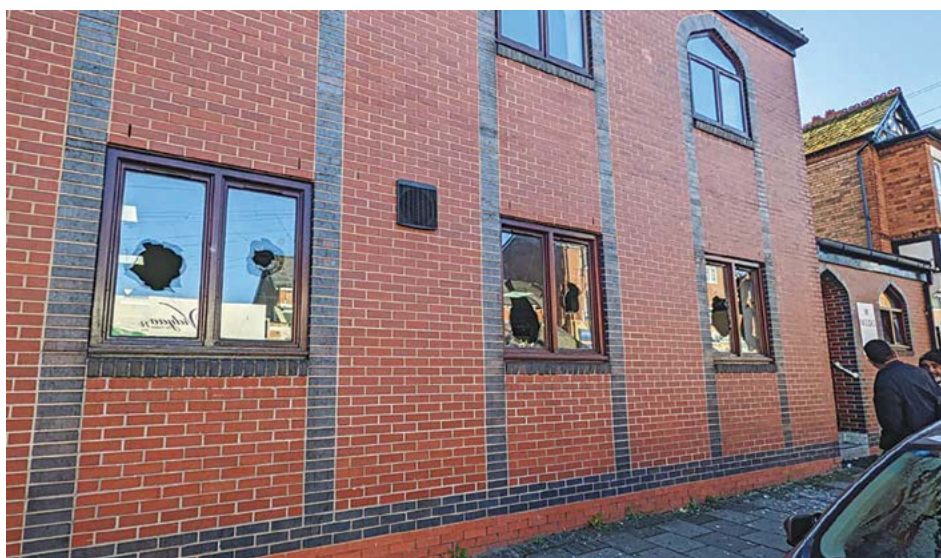
Figure 3: damage to the mosque in Sparkhill, Birmingham caused by the attack 21
